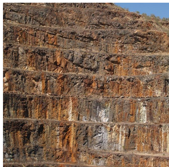
Figure 5 Looking South East final batter showing Rock Fence on the 1000mRL bench and 24m face - 2012
